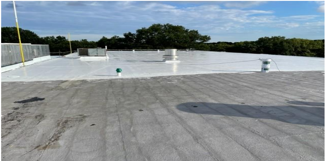
Smithtown High School West new roof Coating is in punch list phase currently
