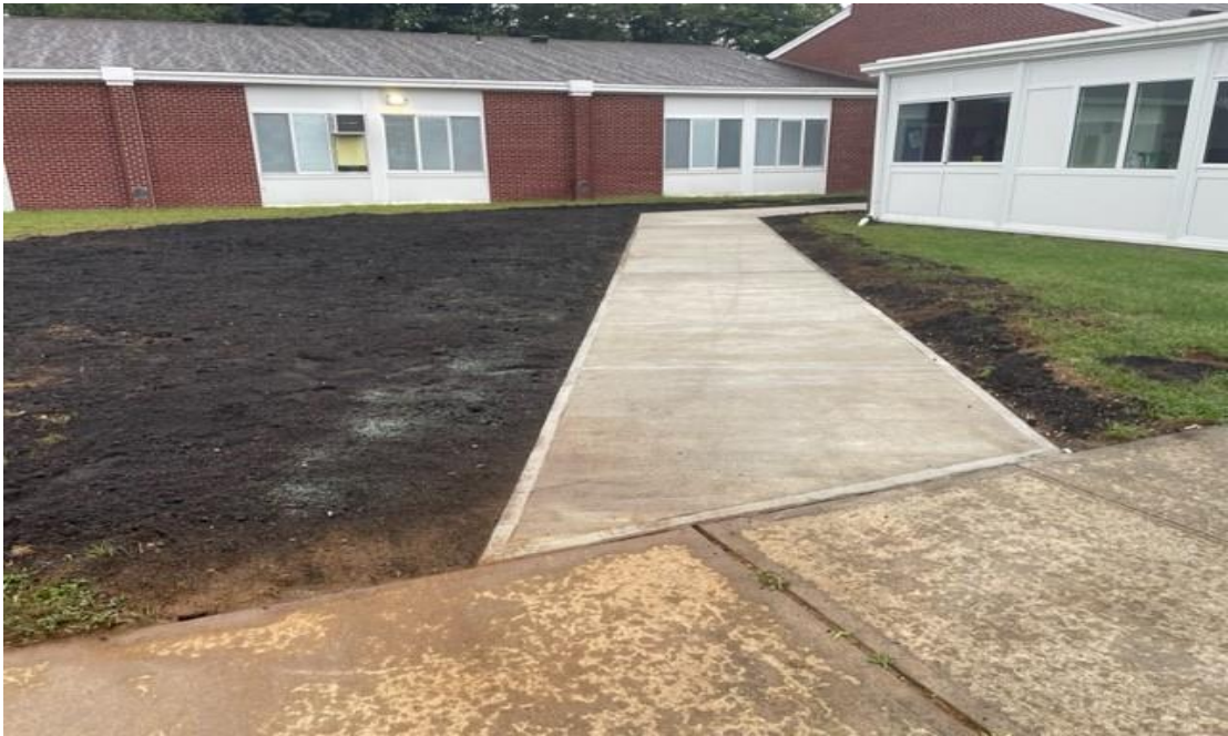
St James Elementary School New Window installation along with repointing around the main Gym and new walkway to new door in corridor behind the multipurpose room
