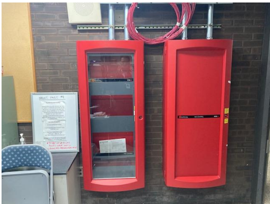
West Fire Alarm – Start and continue installing devices, mount all fire alarm panels
