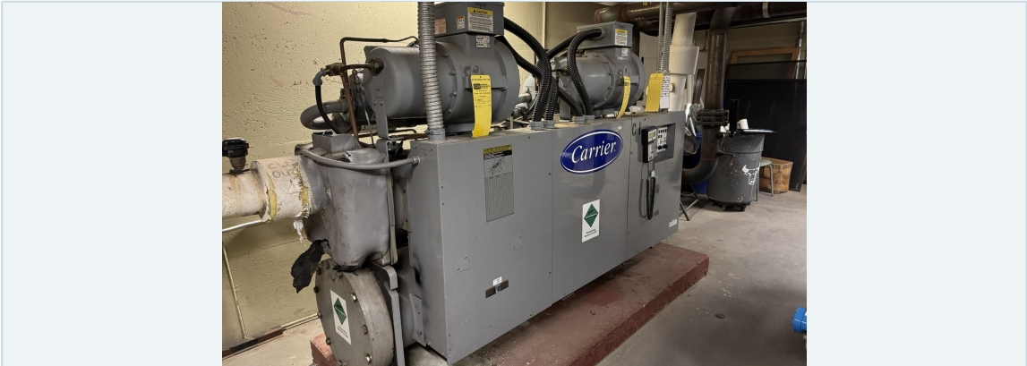
Chiller – High School East
