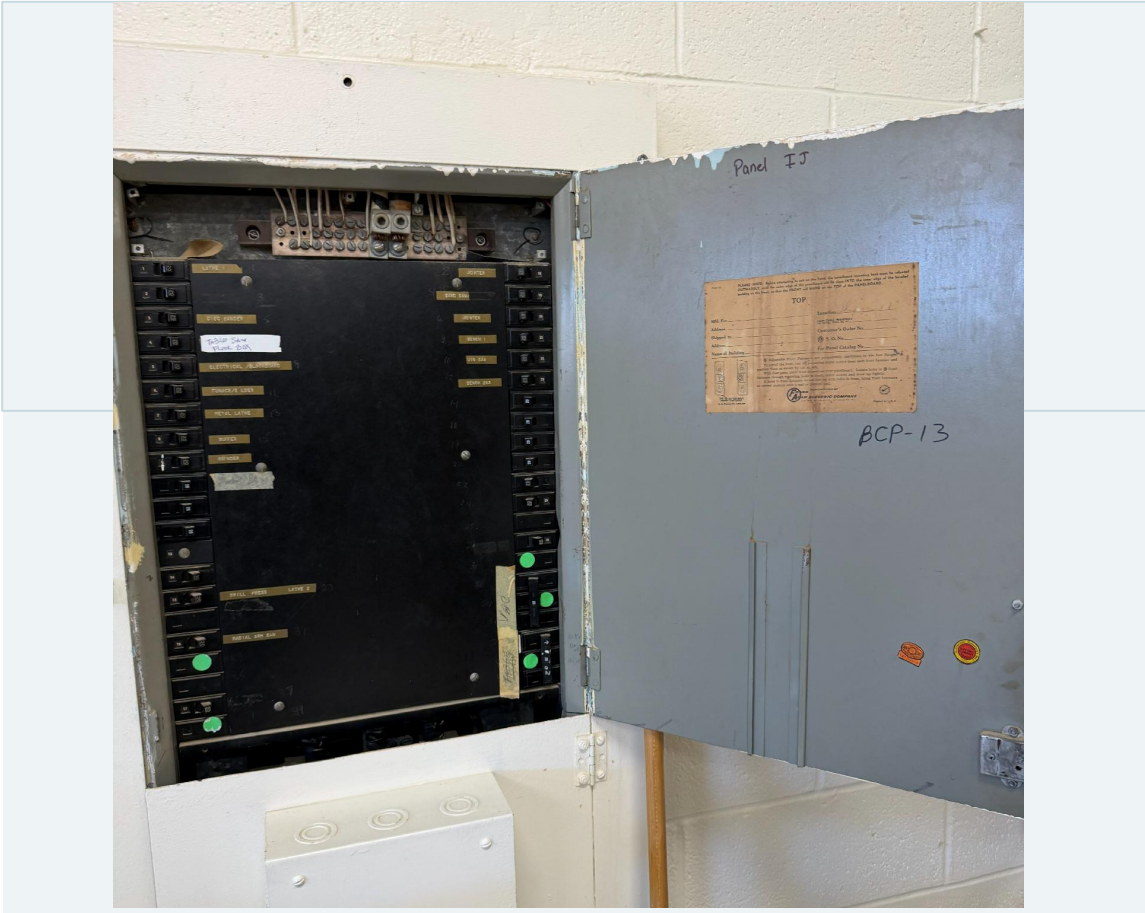
Outdated Electrical Panels
