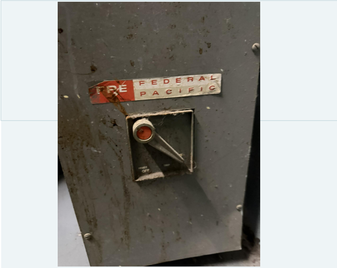
Outdated Electrical Switchgear
