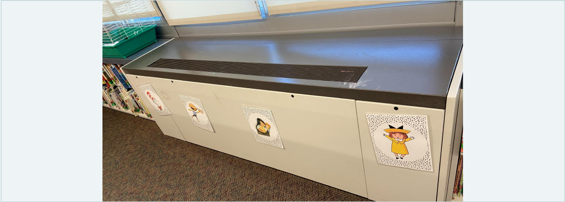
Typical Unit Ventilator – Accomsett Elementary
