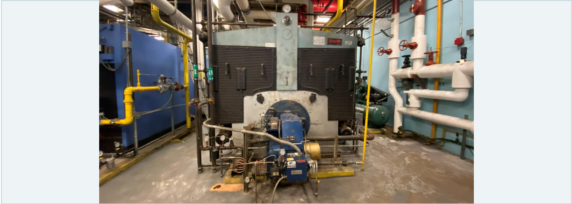
Typical Boiler – High School West
